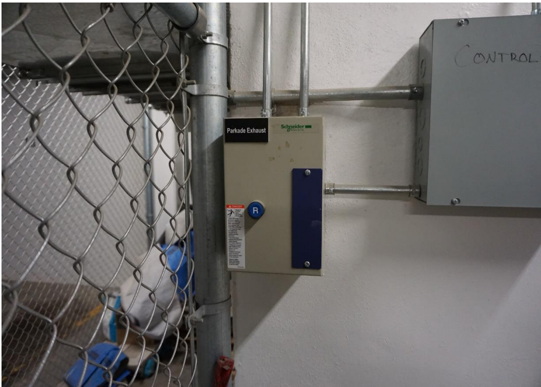
Figure 55 - Parkade exhaust fan controls.
