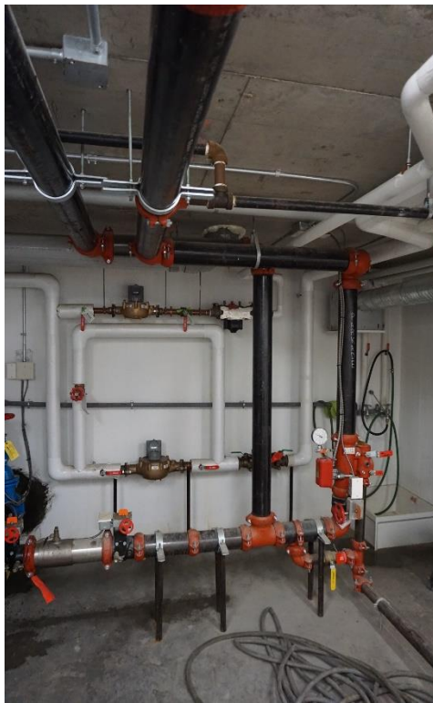
Figure 81 - Fire sprinkler tree.
