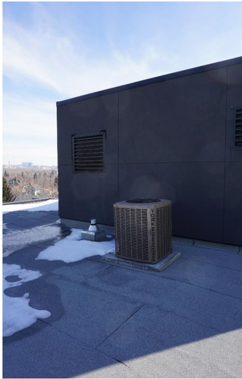
Figure 65 - Hallway MUA condensing unit
