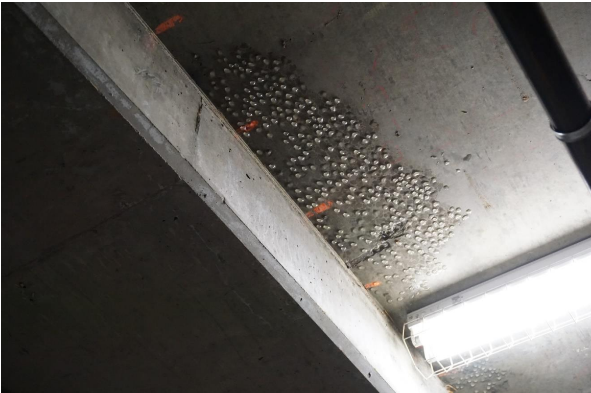
Figure 4 - Condensation on garage ceiling.
