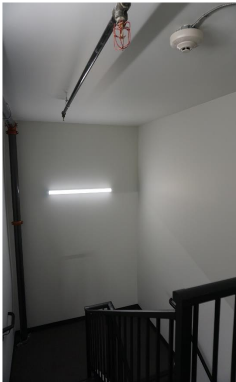
Figure 82 - Fire sprinkler riser, piping, and heads.
