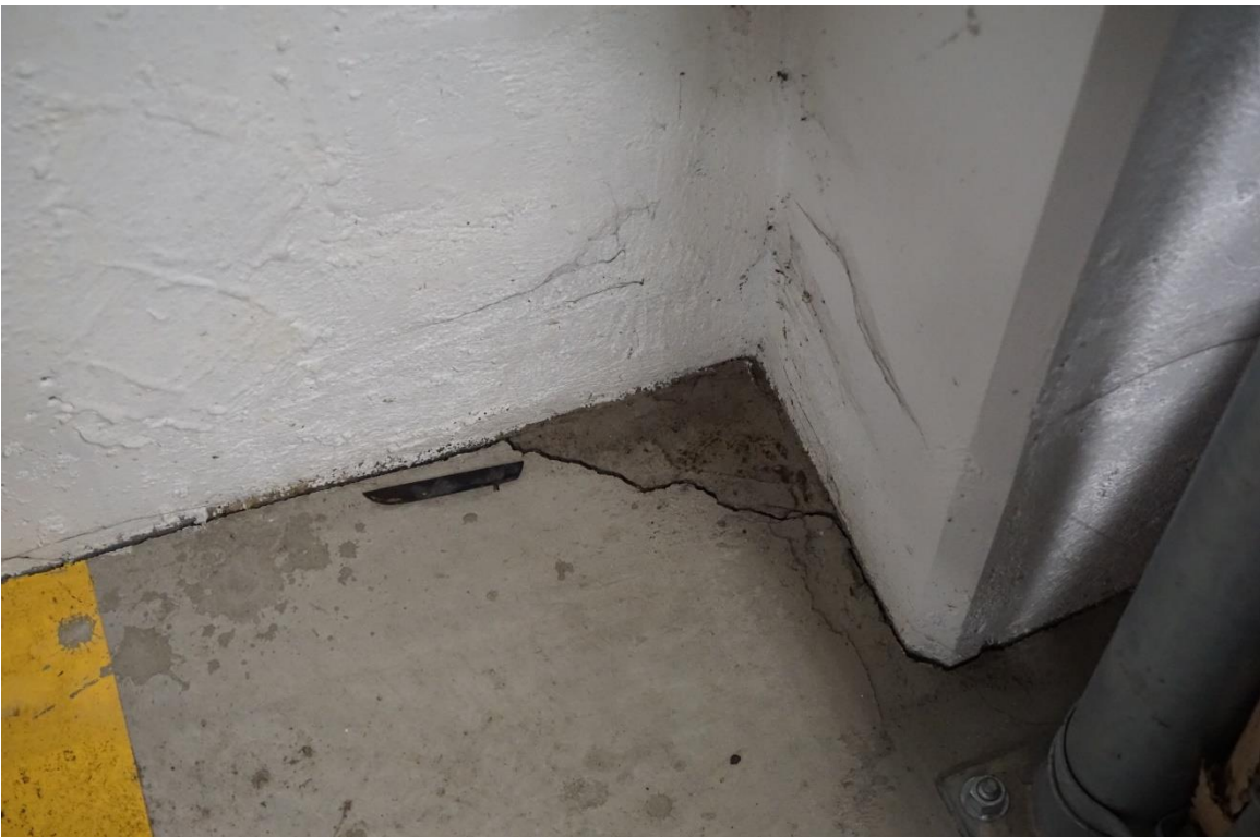
Figure 7 - Minor settlement cracking.
