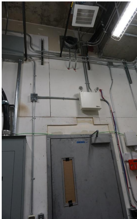
Figure 76 - Emergency lighting battery pack unit.
