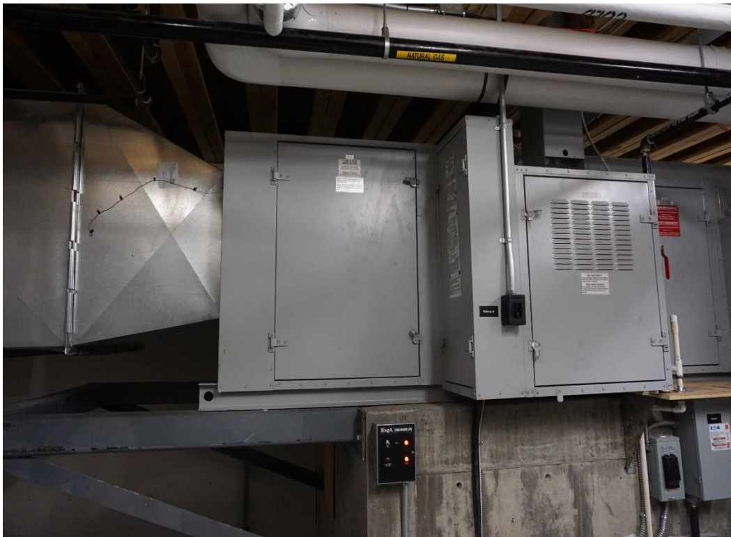
Figure 64 - Engineered Air hallway make-up air unit (MUA).
