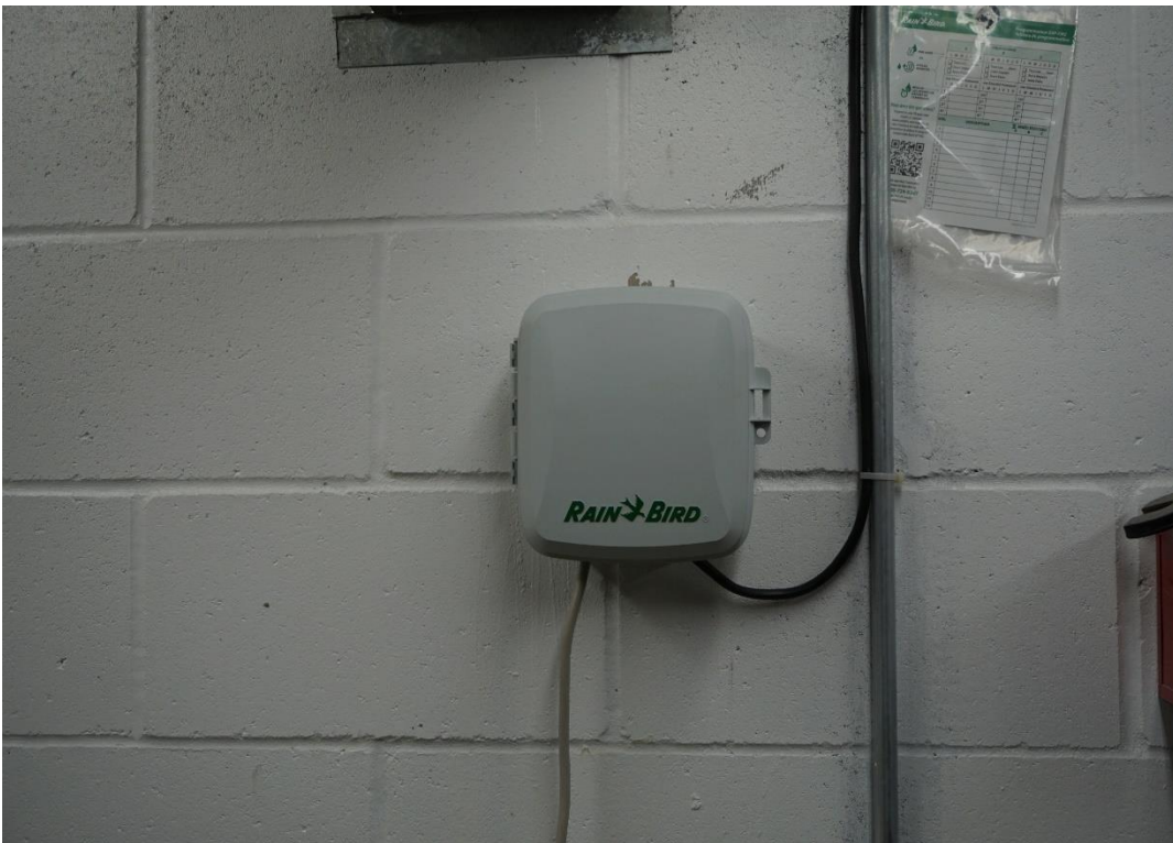
Figure 107 - Irrigation controller located in the parkade water room.
