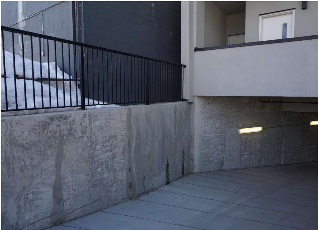
Figure 112 - Concrete retaining wall on the east side of the parkade entrance ramp. Shows some vertical cracking and active leaking.
