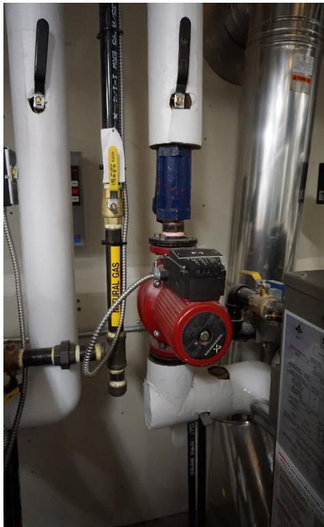
Figure 62 - Boiler recirculating pump (P-3).
