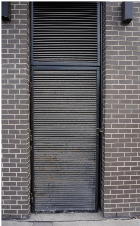
Figure 17 - Louvered metal gas room door.
