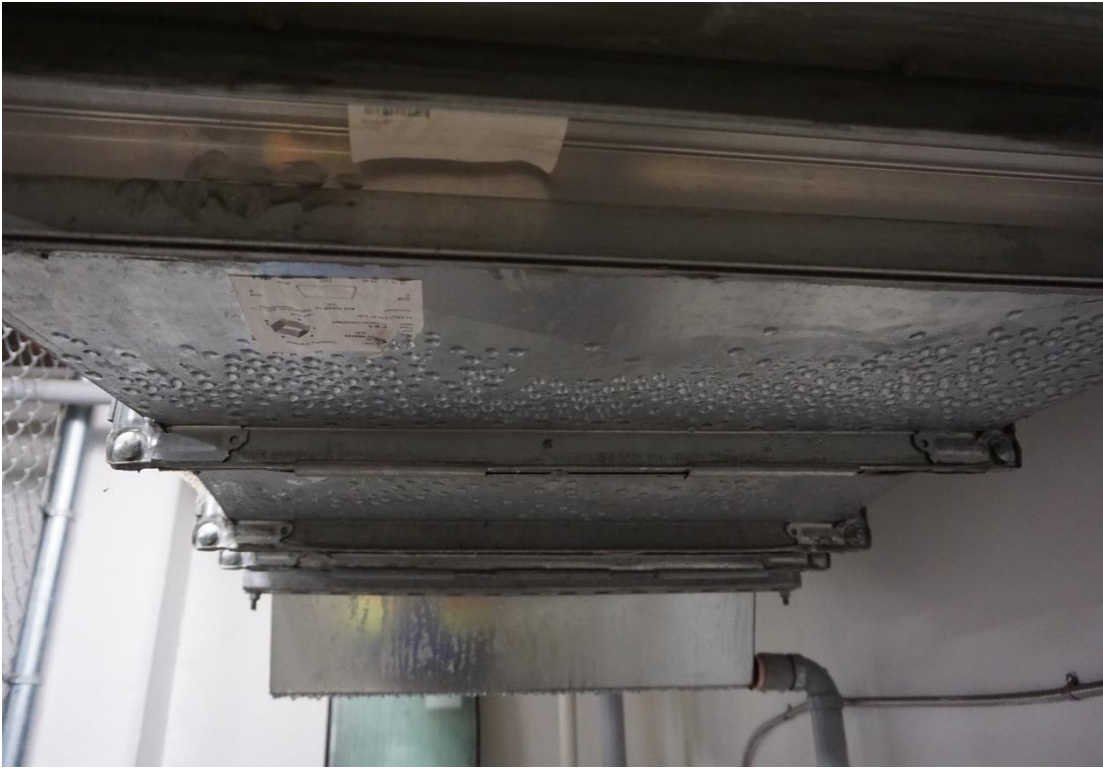
Figure 56 - Condensation on the underside of the parkade exhaust fan.
