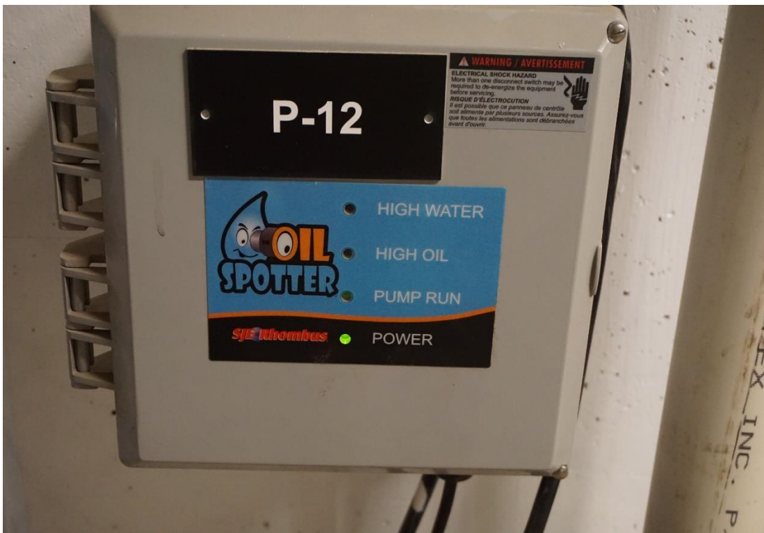
Figure 73 - Controller for the elevator sump pump.
