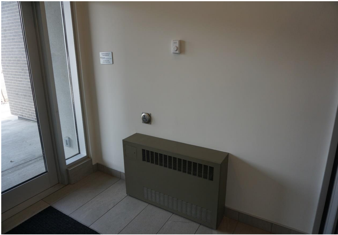
Figure 60 - Force flow heater in the front entrance vestibule.
