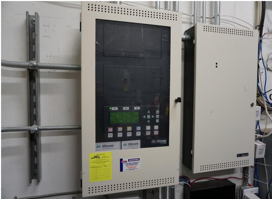
Figure 78 - Fire alarm panel.
