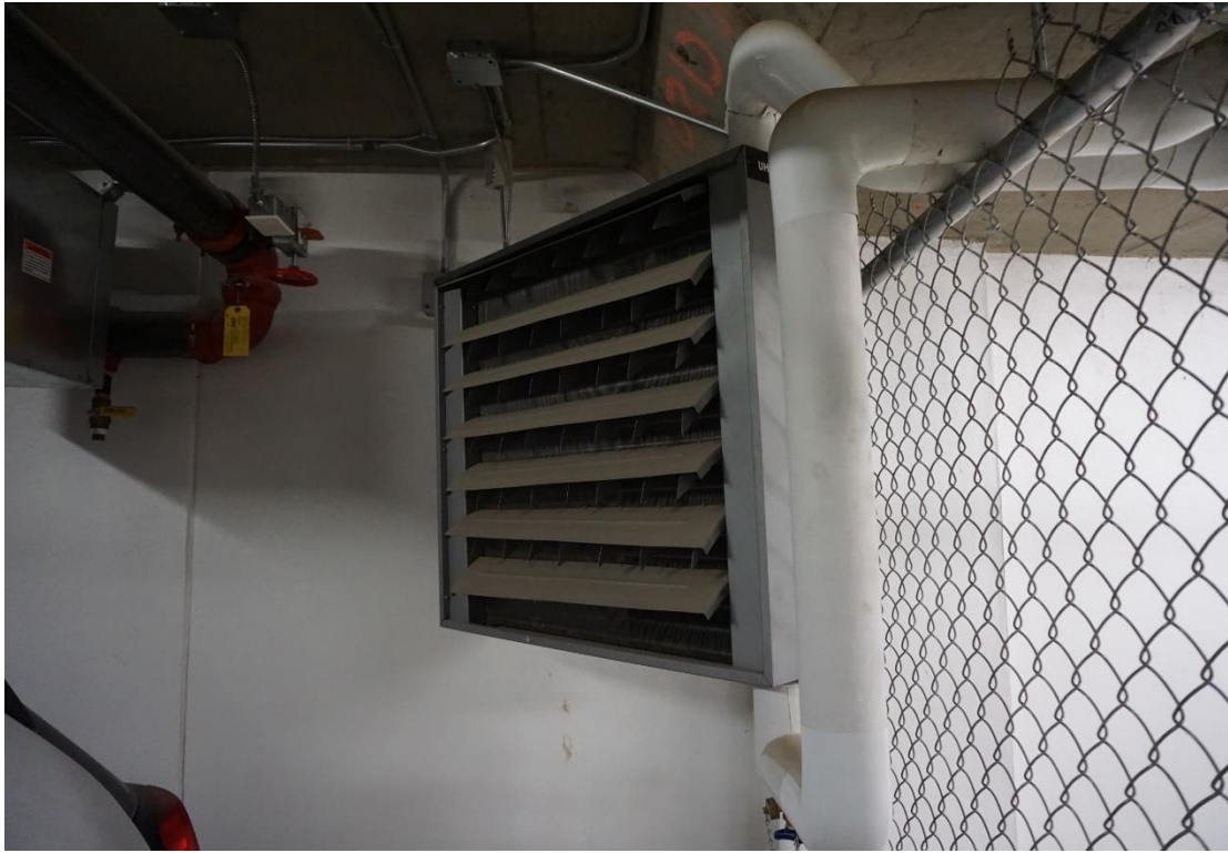
Figure 61 - Hydronic unit heater in the parkade.
