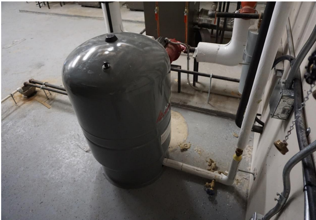
Figure 59 - Expansion tank for the commercial boiler.
