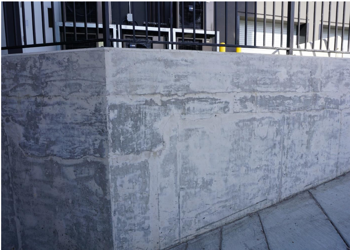
Figure 113 - Concrete retaining wall on the west side of the parkade entrance ramp. Shows long horizontal crack.
