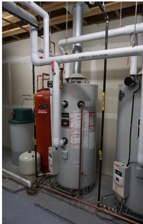
Figure 58 - Expansion tank for the residential boilers (red tank).
