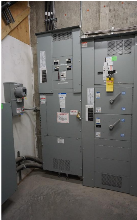
Figure 41 - Main distribution panel with disconnects.
