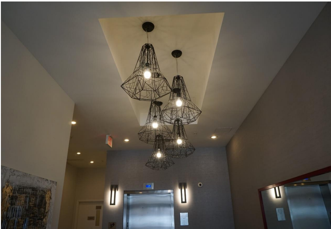
Figure 39 - Pendant, wall sconce and recessed pot lights in the main lobby.
