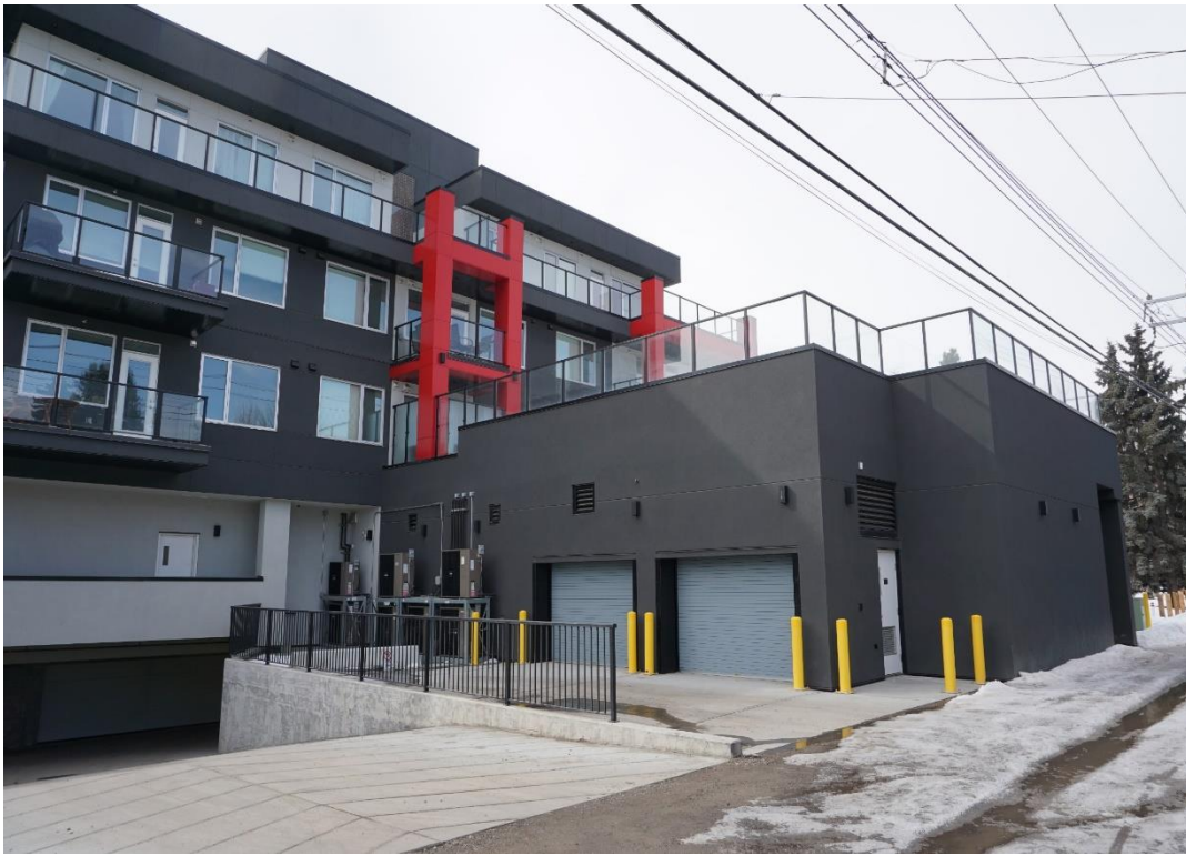
Figure 104 - Concrete elements including the parkade ramp, loading area and jersey barrier. Also shows the retaining wall.
