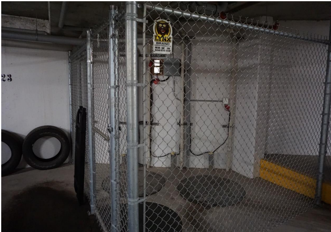
Figure 72 - Sump cage with three basin covers. The sump pumps are located at the bottom of the basins.
