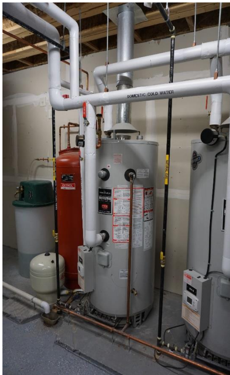
Figure 50 - Chemical mix tank (clear tank with green top) and the domestic hot water expansion tank (small cream-colored tank).
