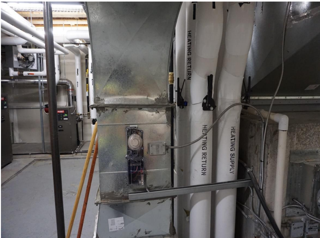
Figure 49 - 500 MBH boiler servicing the commercial units.
