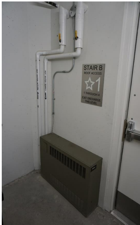
Figure 63 - Insulated hot water supply and return lines.
