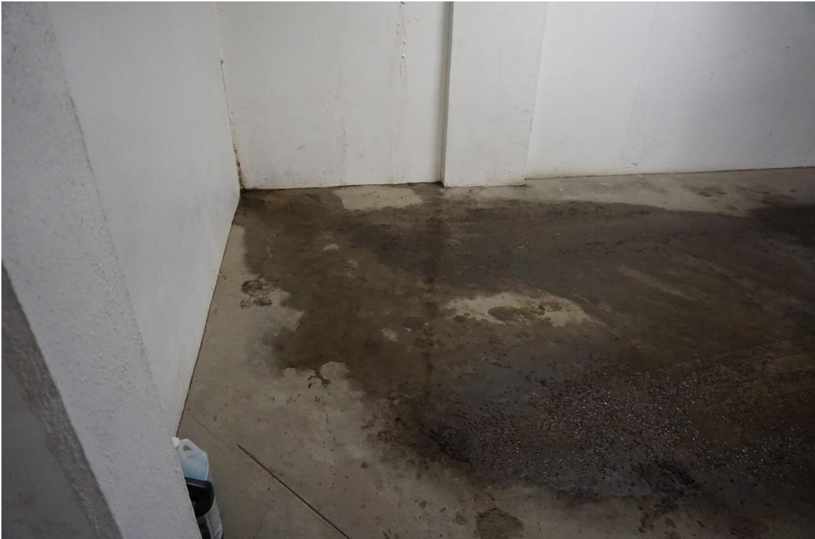
Figure 2 - Leaking from wall and onto slab.
