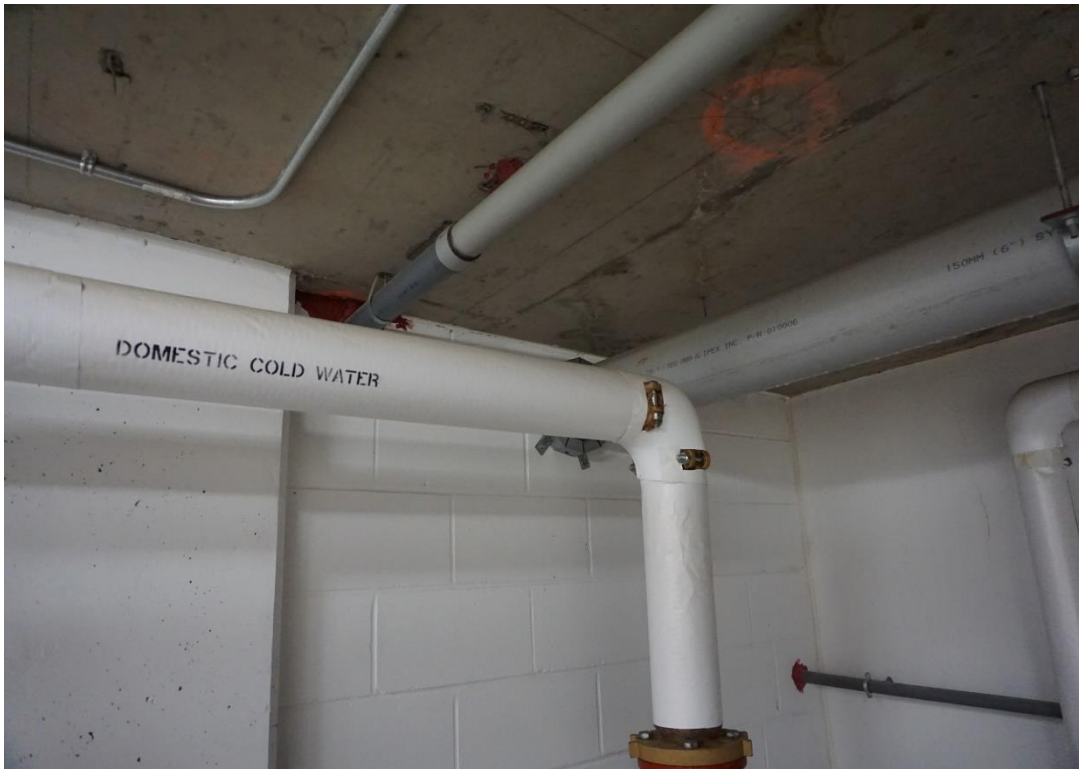
Figure 67 - Insulated domestic cold-water lines.
