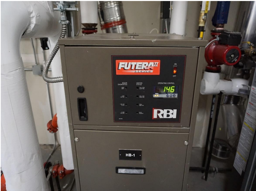
Figure 48 - One of two 1000 MBH heating boilers.
