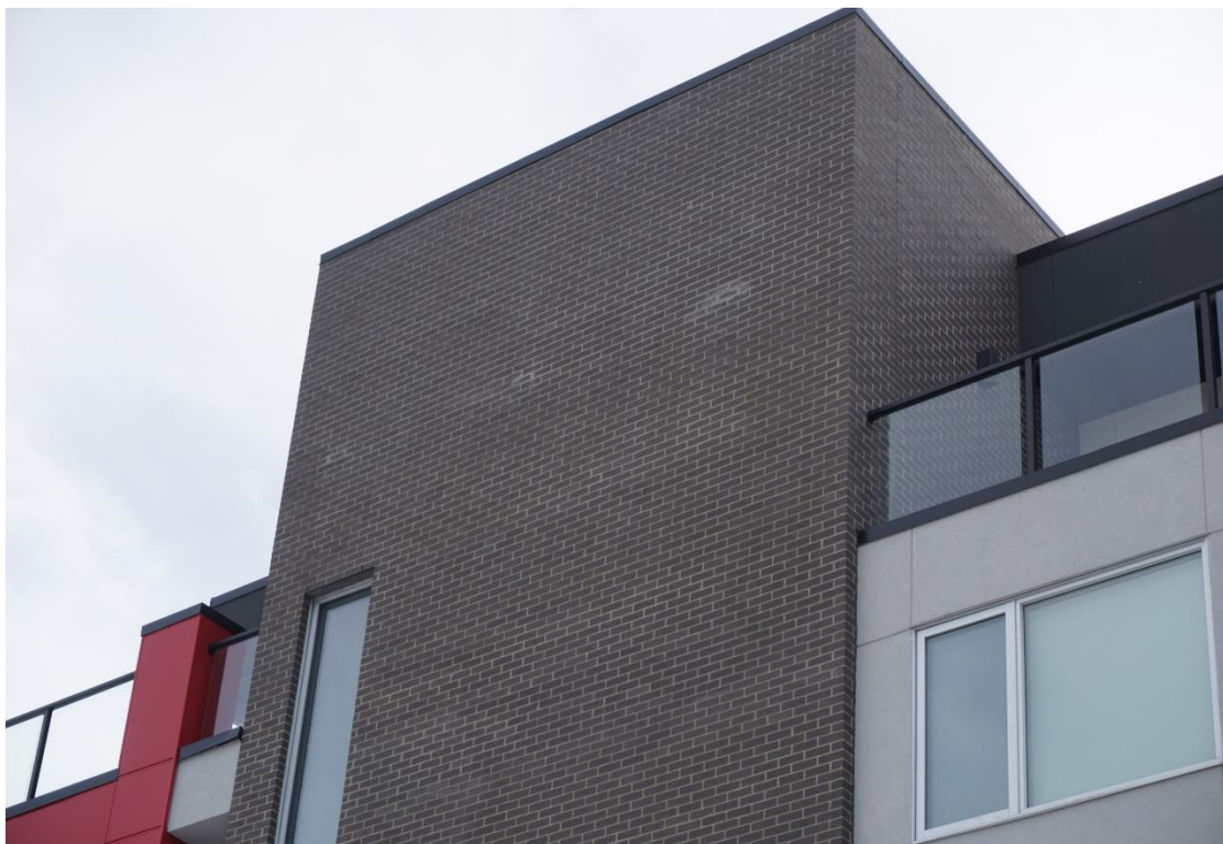
Figure 12 - Some efflorescence on the bricks on the west side stairwell.
