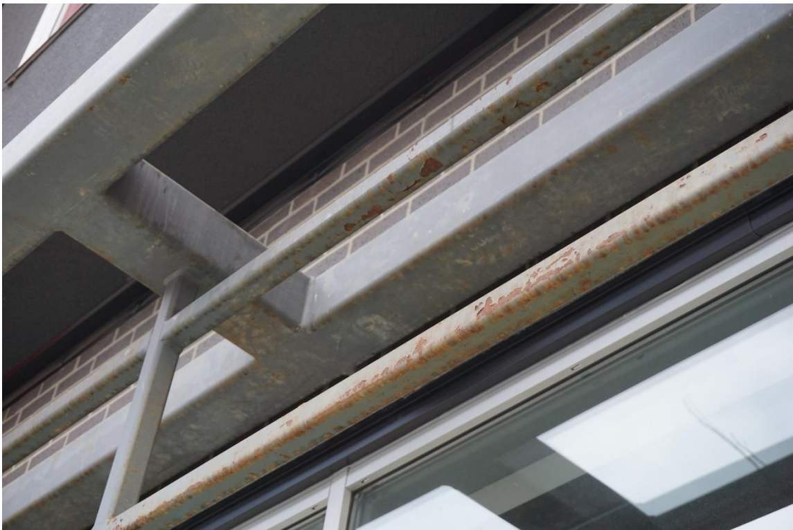
Figure 9 - Condition during our first visit. Top coating over this steel will not yield good results. Proper preparation must be done.
