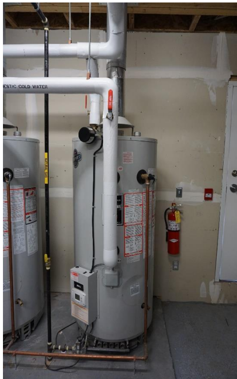
Figure 52 - Bradford White domestic hot water tanks.
