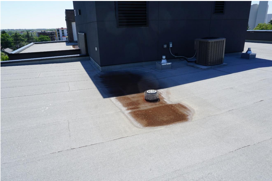
Figure 32 - Roof over 4th floor. Standing water present approaching the 48 hour mark.
