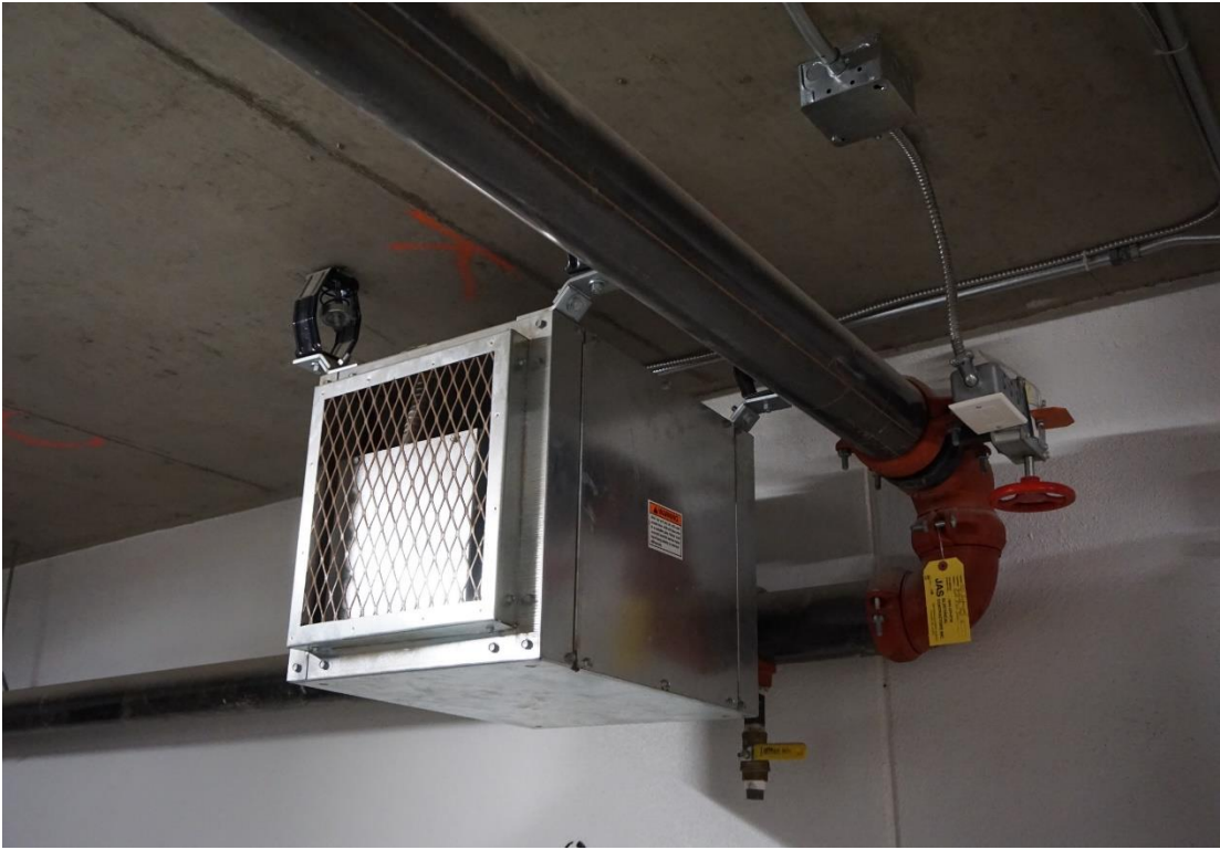
Figure 57 - One of three parkade transfer fans.
