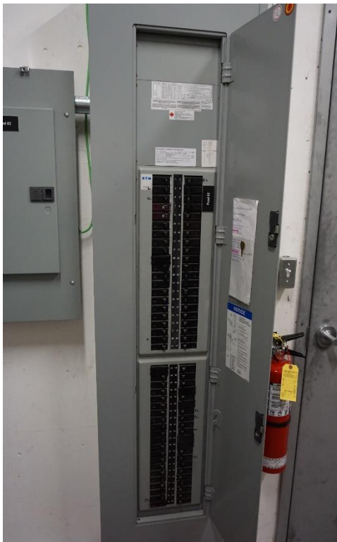
Figure 43 - Main house panel.
