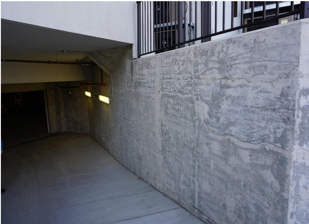
Figure 35 - Wall mounted fluorescent lighting on the parkade ramp.
