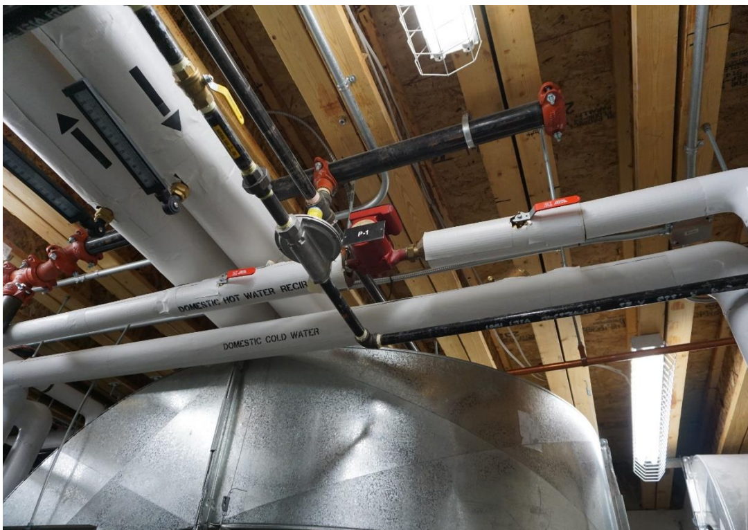
Figure 53 - Domestic hot water recirculation pump (P-1) and insulated hot and cold-water lines.
