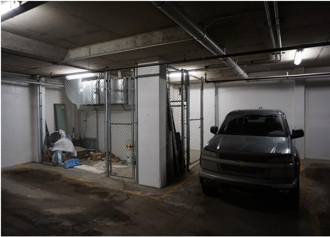
Figure 54 - Parkade exhaust fan.
