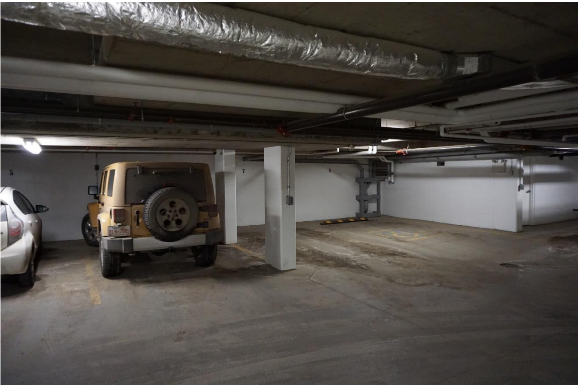
Figure 6 - Note the white salt staining on the slab.
