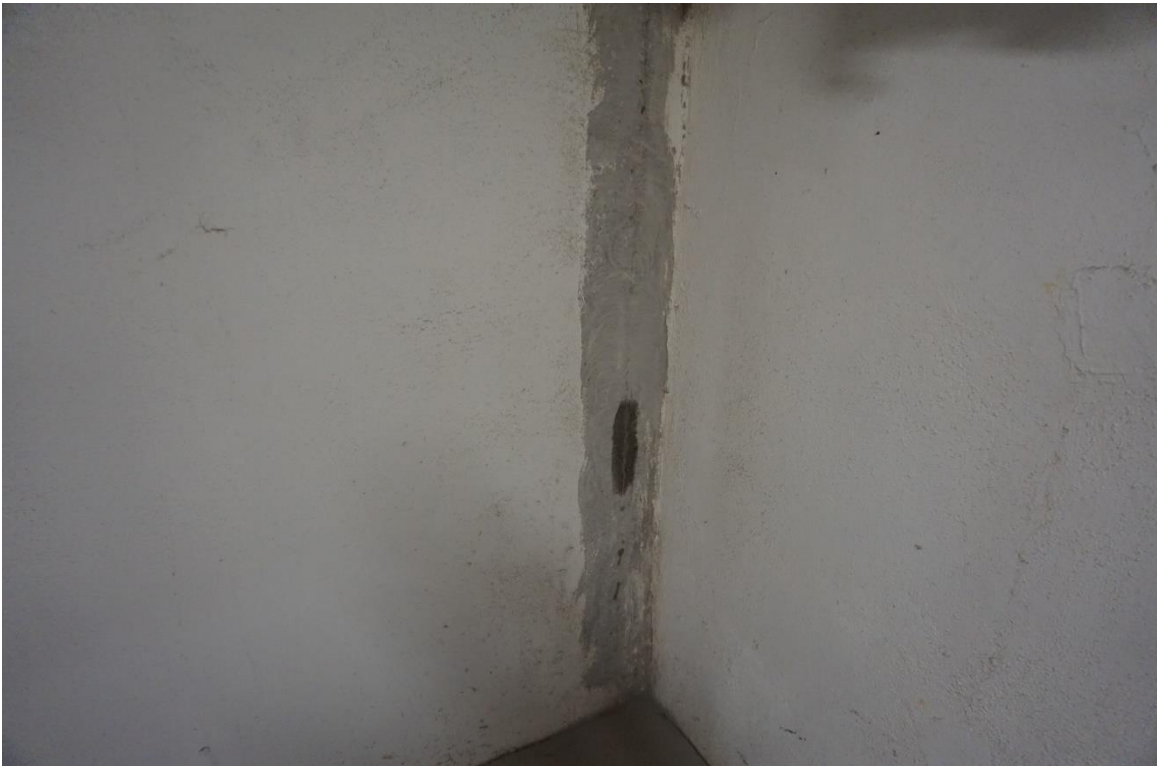
Figure 3 - Leak patched but still leaking.
