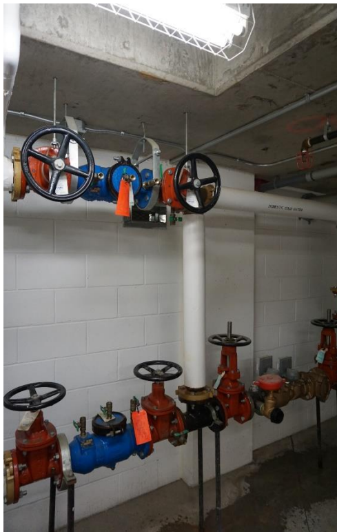
Figure 46 - Two domestic water system backflow prevention devices.
