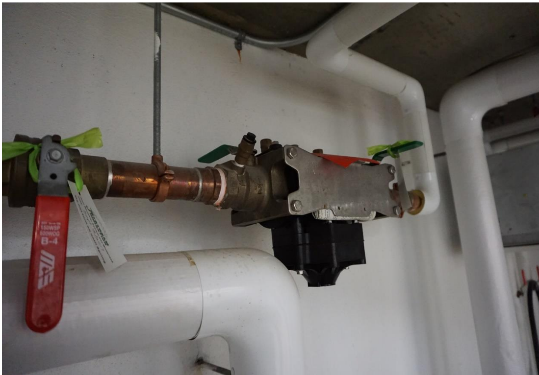
Figure 47 - Irrigation system backflow prevention device.
