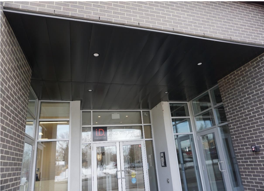
Figure 34 - Recessed LED pot lights at the front entrance.
