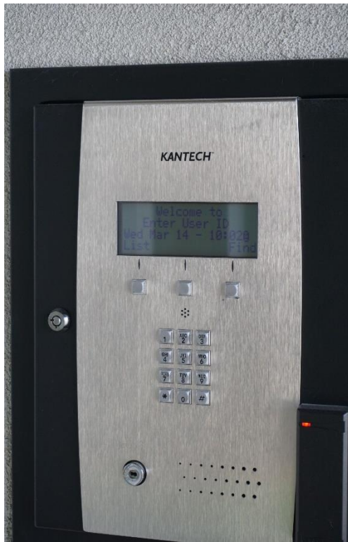
Figure 36 - Intercom system and access card reader.
